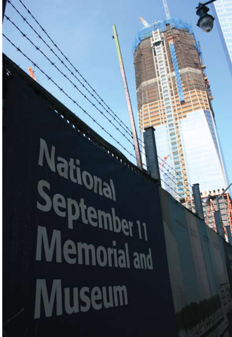
Construction continued at One World Trade Center, formerly known as the Freedom Tower, on May 7.
